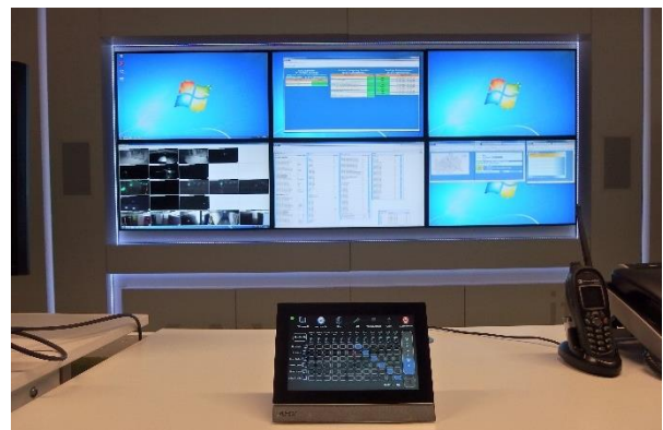
Videowall and touch screen panel in control room
