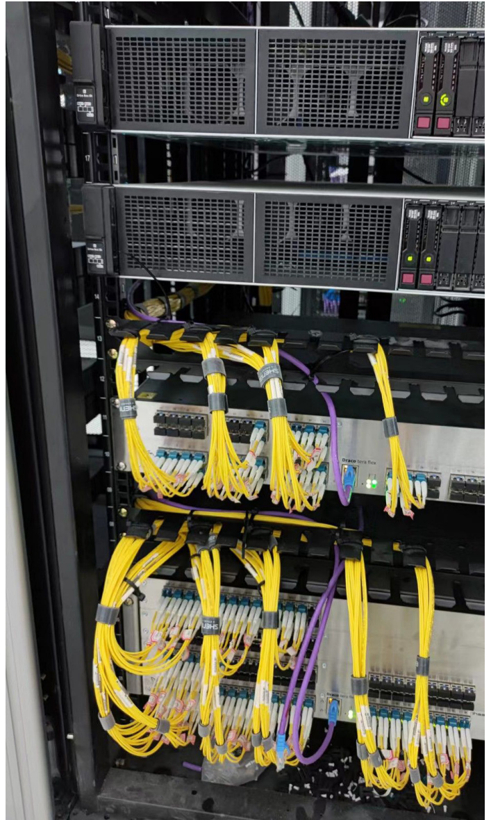
Draco tera flex matrix switches in operation
